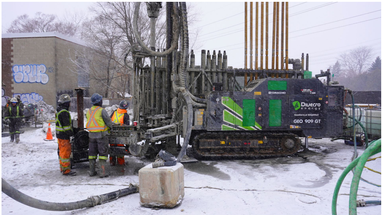
Courtesy of the Ontario Geothermal Association
