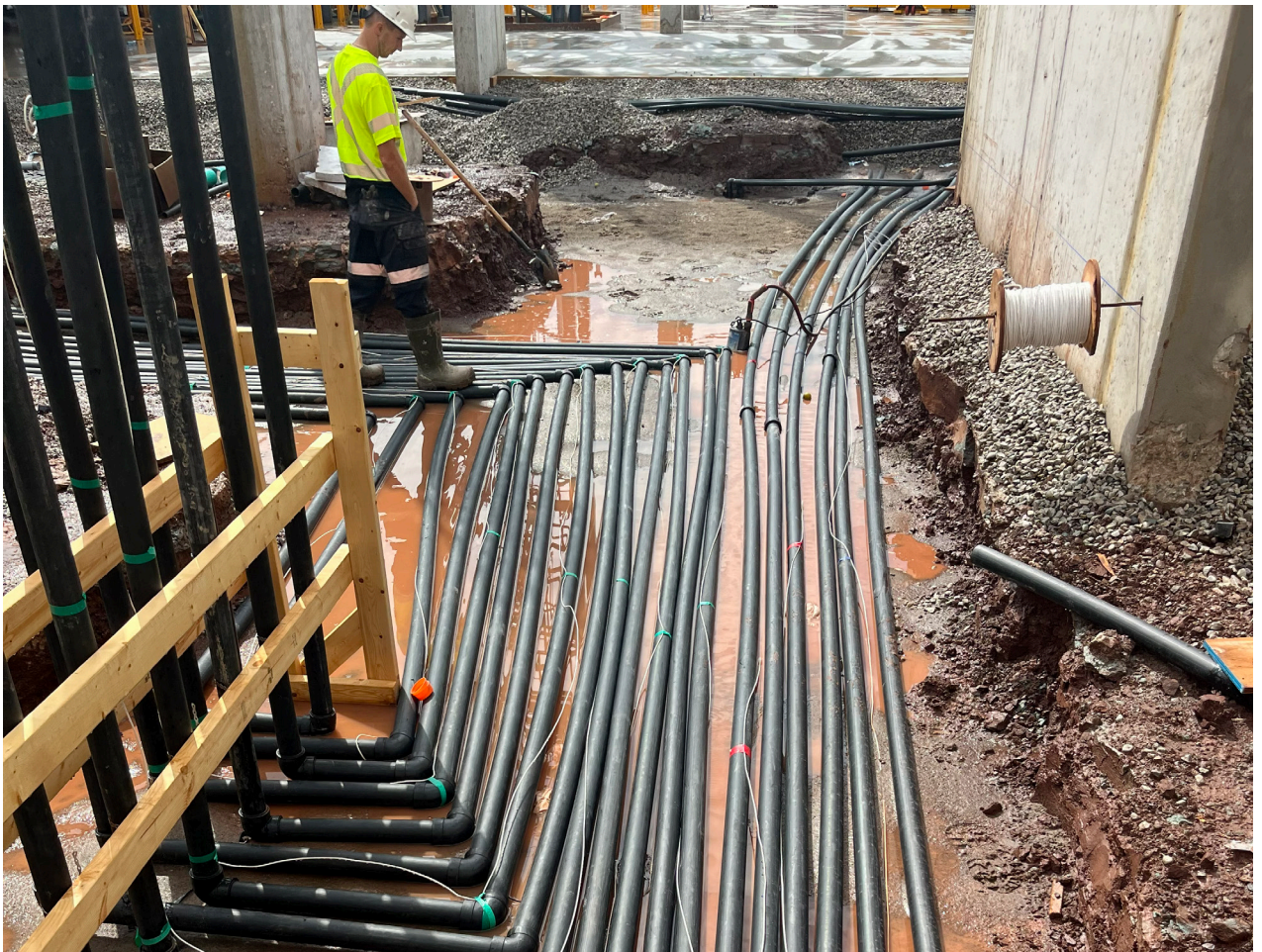
Courtesy of the Ontario Geothermal Association
